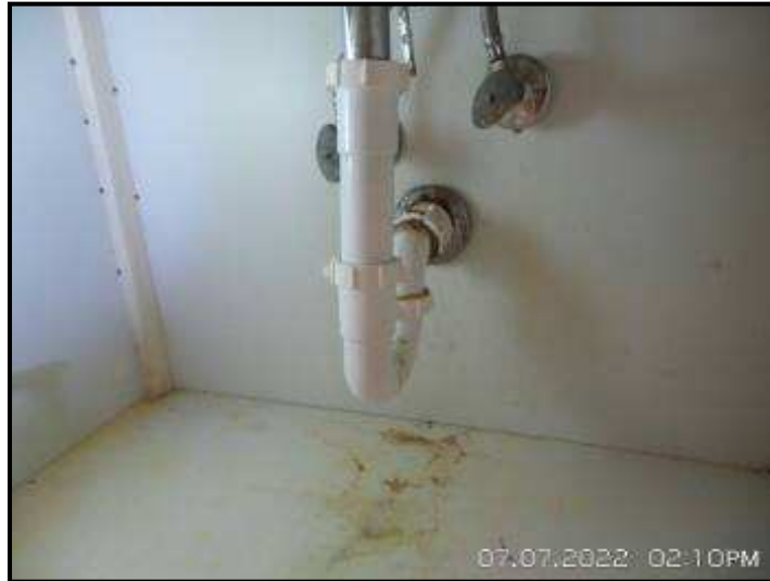
Drain line leaks under sink.
