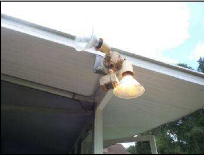
Damaged light fixtures observed.
