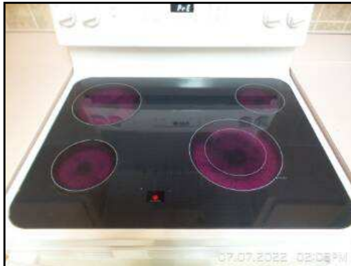
All heating elements operated when tested.
