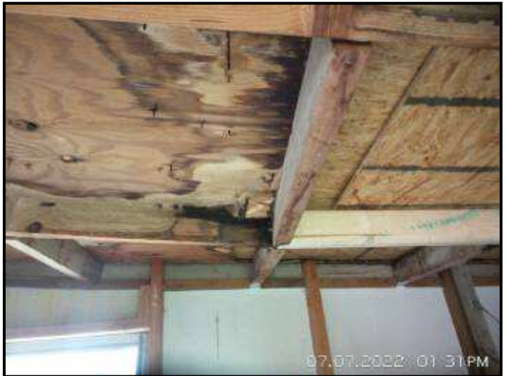
Exterior closet that contains the water treatment system shows signs of significant wood rot. It appears to be near the end of its useful life. Recommend replacement.
