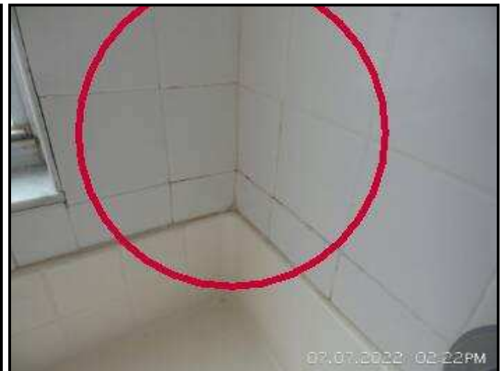
Loose tiles noted. Recommend review by a licensed contractor for repair or replacement.
