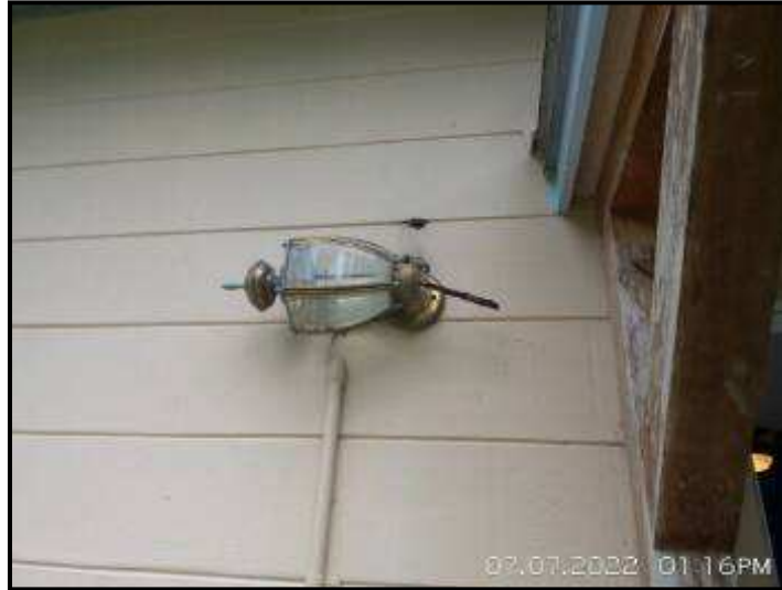
Damaged light fixtures observed.
