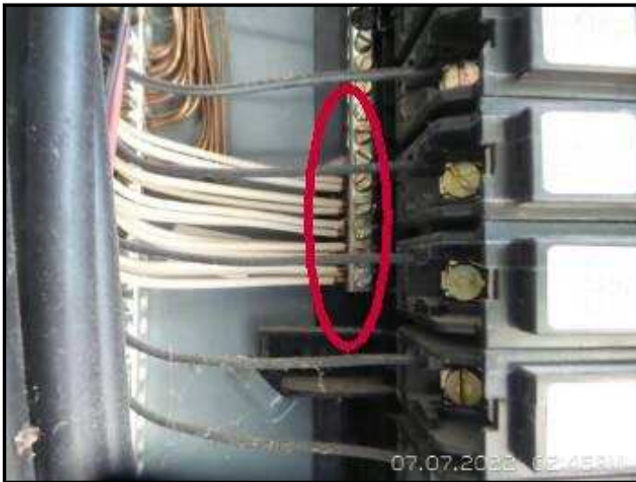
Double tapped connections inside panel box (more than one electrical conductor attached to a single screw and/or lug). This is not standard practice, and may cause overheating or even an electrical fire. Recommend evaluation by an electrician.
