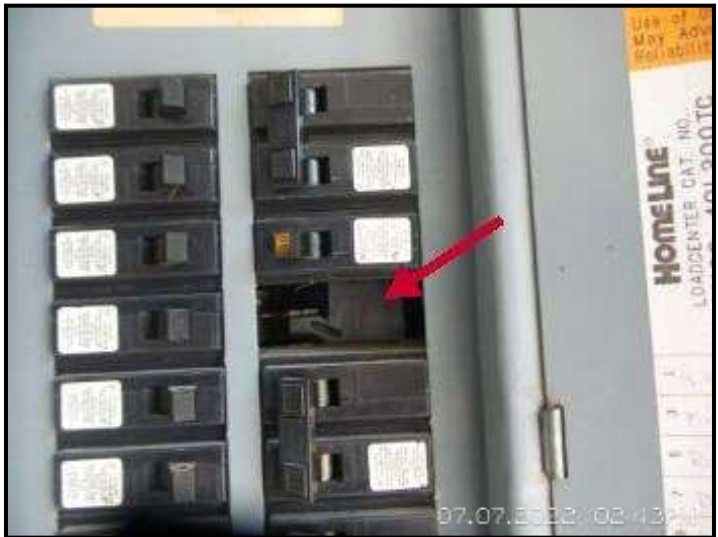
Open breaker panel slot(s) at panel box cover. Electrocutation hazard.
