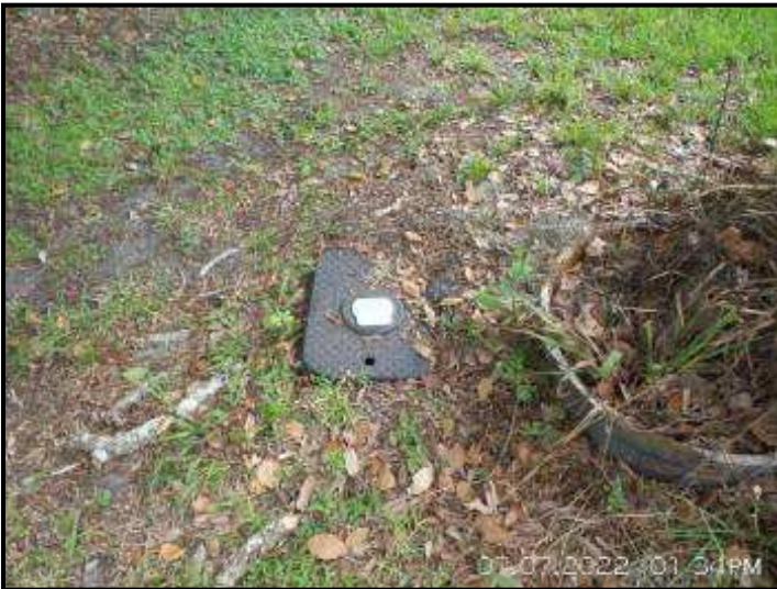
Main water shut off is in the meter box at the street
