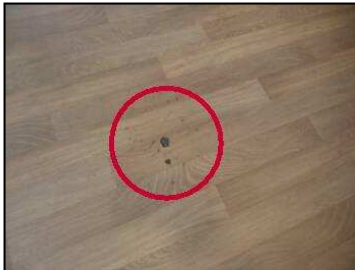
Minor damage noted.
