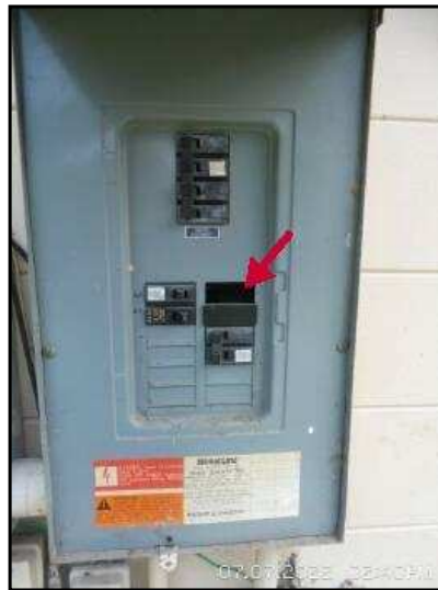
Open breaker panel slot(s) at panel box cover. Electrocutation hazard.
