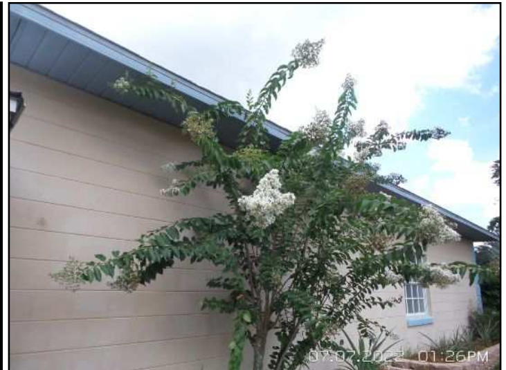
Prune or remove any plants that are in contact or proximity to home to eliminate pathways of wood destroying insects.
