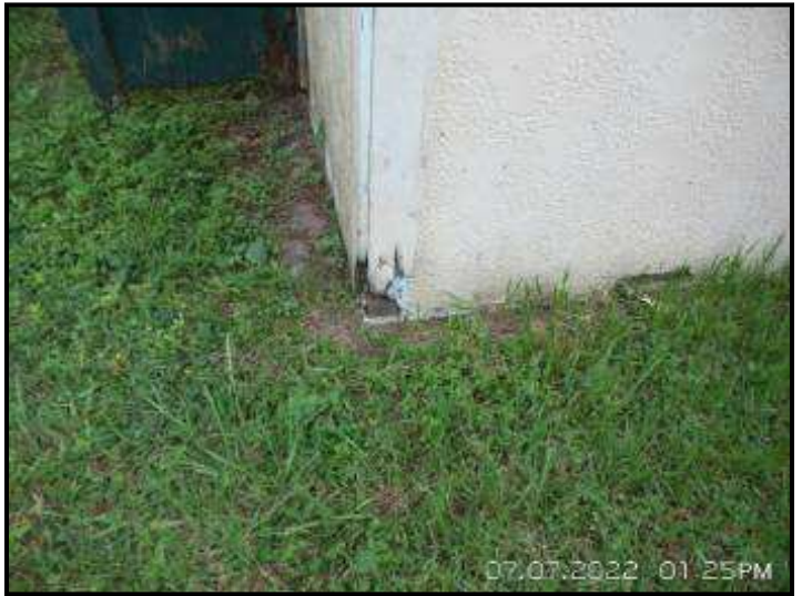
Exterior closet that contains the water treatment system shows signs of significant wood rot. It appears to be near the end of its useful life. Recommend replacement.
