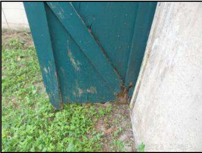
Exterior closet that contains the water treatment system shows signs of significant wood rot. It appears to be near the end of its useful life. Recommend replacement.
