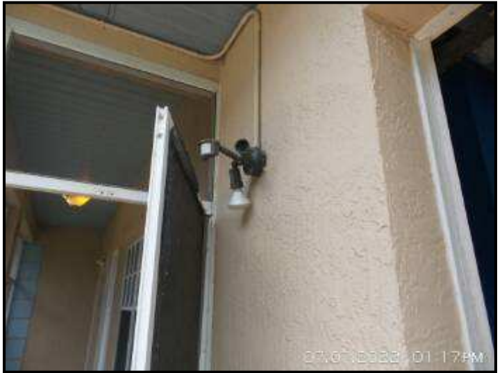
Damaged light fixtures observed.
