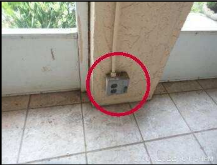
Outlet at the front porch did not have power.
