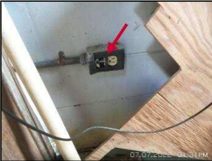
Damaged electrical outlet observed in the exterior closet.
