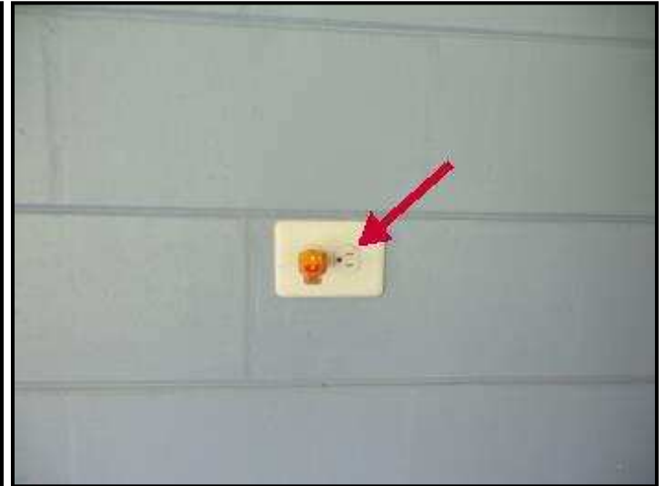
Reversed polarity, hot and neutral reversed and other terms used for electric receptacles are usually easily corrected by minor wiring adjustments at the specified item. When these conditions are noted in this report, a licensed electrician should be consulted for repairs/replacement as needed to ensure safety.
