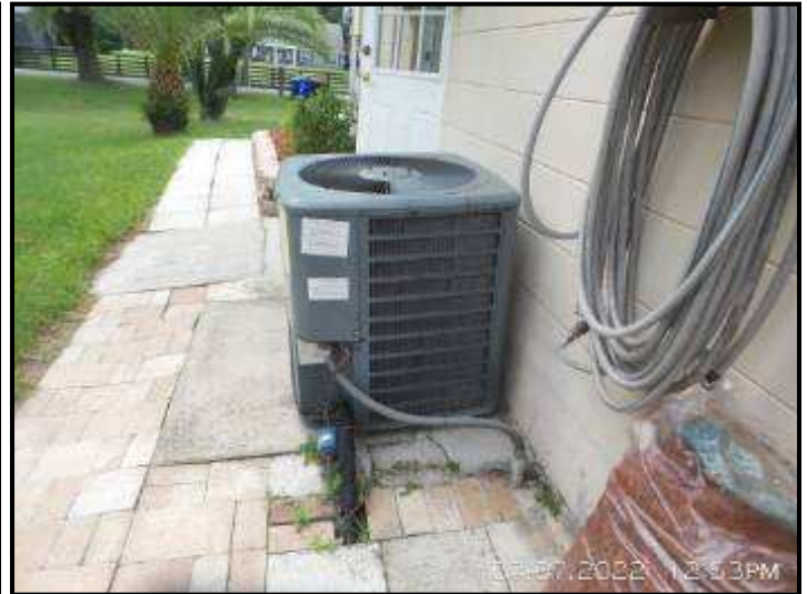
Exterior unit not level. This can affect system performance.
