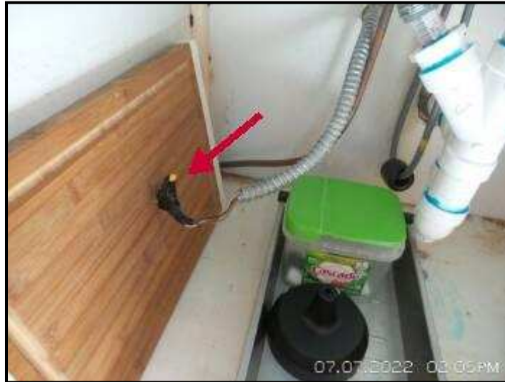
Exposed wiring observed under the sink.
