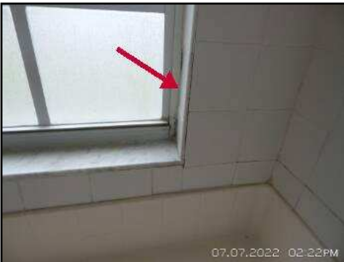
Loose tiles noted. Recommend review by a licensed contractor for repair or replacement.
