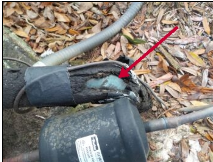
Missing insulation at A/C unit.
