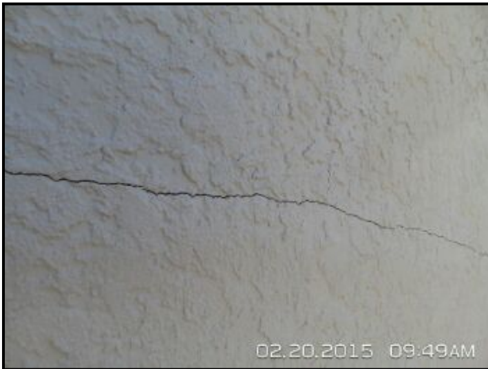
Cracking observed at several areas around home. Appears to have been repaired once already and has cracked again. This is a sign of possible continuous movement. Cracking of this type is possible source of moisture entering into the walls. Recommend licensed contractor evaluate and make recommendations for repairs.
