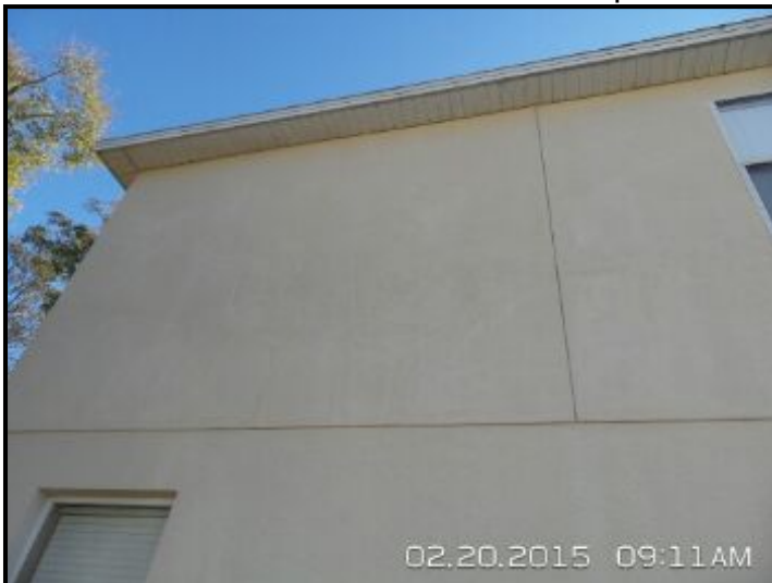
Cracking observed at several areas around home. Appears to have been repaired once already and has cracked again. This is a sign of possible continuous movement. Cracking of this type is possible source of moisture entering into the walls. Recommend licensed contractor evaluate and make recommendations for repairs.
