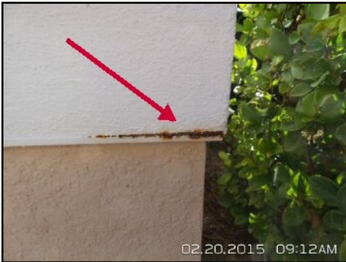
Areas of stucco show rust and deterioration of underlying metal corners. This is a sign of possible moisture in the wall space. Recommend licensed contractor evaluate and make recommendations for repairs.
