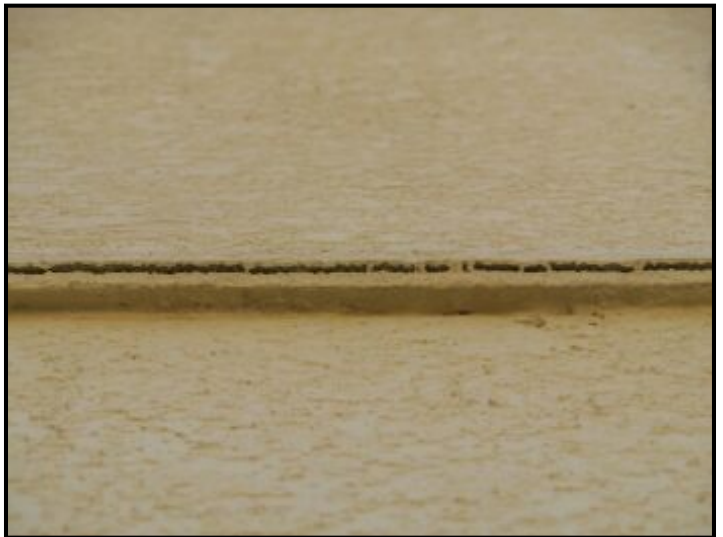
Cracking observed at several areas around home. Appears to have been repaired once already and has cracked again. This is a sign of possible continuous movement. Cracking of this type is possible source of moisture entering into the walls. Recommend licensed contractor evaluate and make recommendations for repairs.
