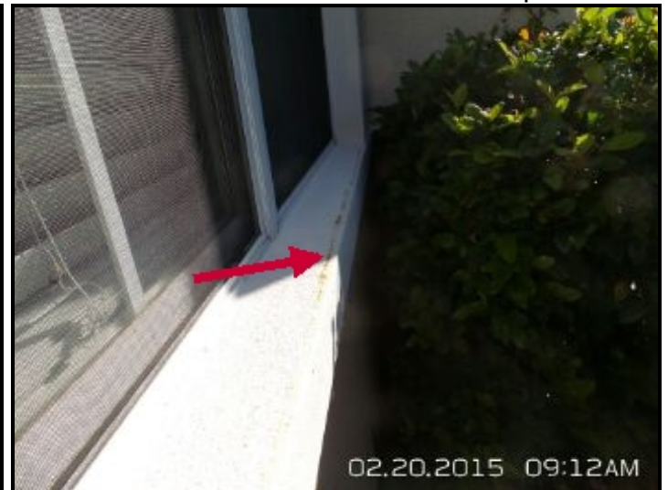
Areas of stucco show rust and deterioration of underlying metal corners. This is a sign of possible moisture in the wall space. Recommend licensed contractor evaluate and make recommendations for repairs.
