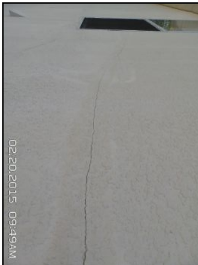
Cracking observed at several areas around home. Appears to have been repaired once already and has cracked again. This is a sign of possible continuous movement. Cracking of this type is possible source of moisture entering into the walls. Recommend licensed contractor evaluate and make recommendations for repairs.
