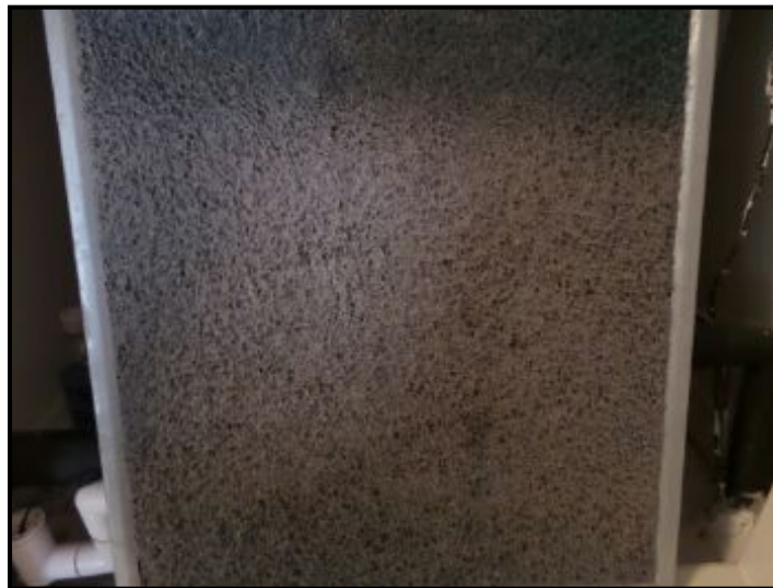
Filter dirty. Needs replacement.
