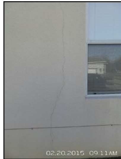
Cracking observed at several areas around home. Appears to have been repaired once already and has cracked again. This is a sign of possible continuous movement. Cracking of this type is possible source of moisture entering into the walls. Recommend licensed contractor evaluate and make recommendations for repairs.
