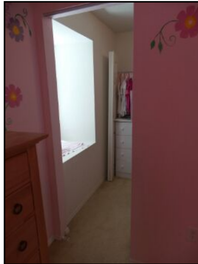
Closet door has fallen off.
