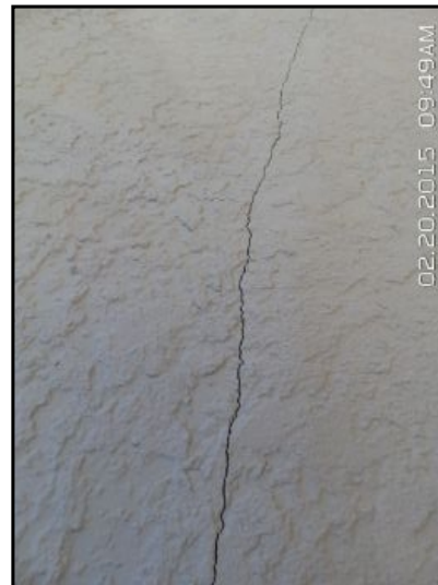
Cracking observed at several areas around home. Appears to have been repaired once already and has cracked again. This is a sign of possible continuous movement. Cracking of this type is possible source of moisture entering into the walls. Recommend licensed contractor evaluate and make recommendations for repairs.
